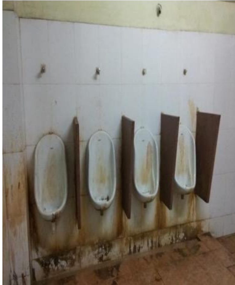
Urinal not clean
