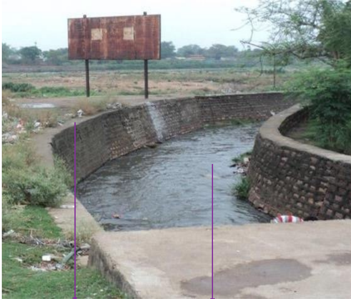
Boundary wall Nallah Without Solid Waste Floating
