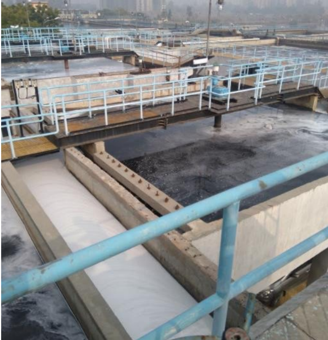
Photograph of STP plant
