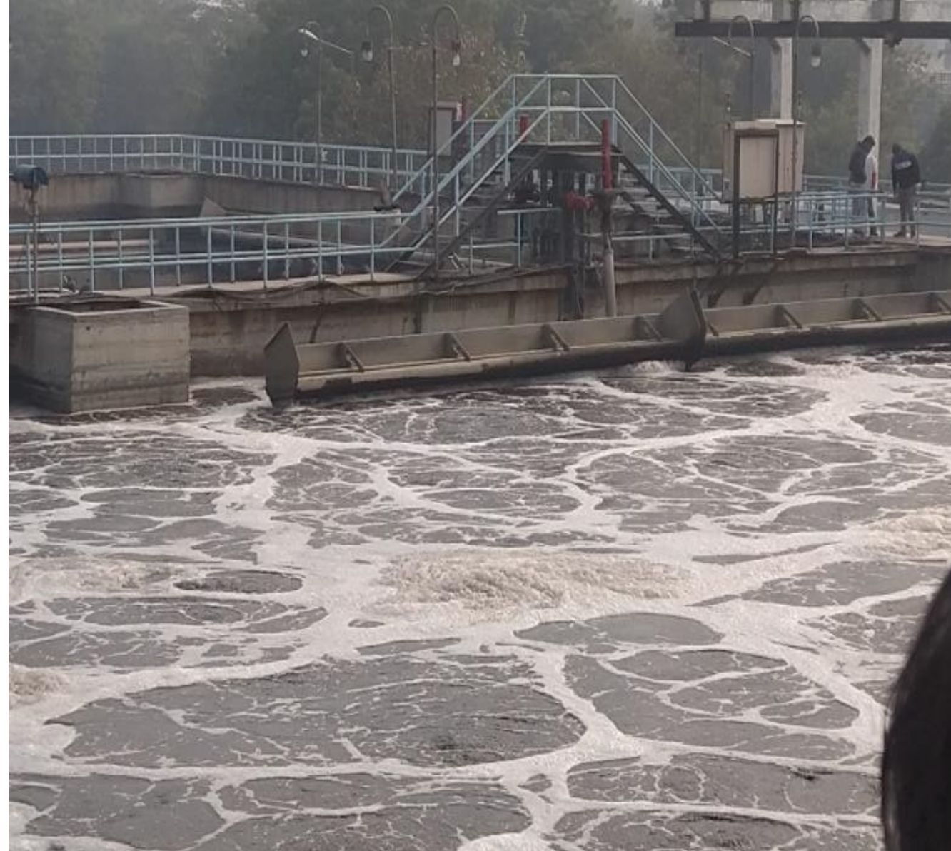
Photograph of STP plant
