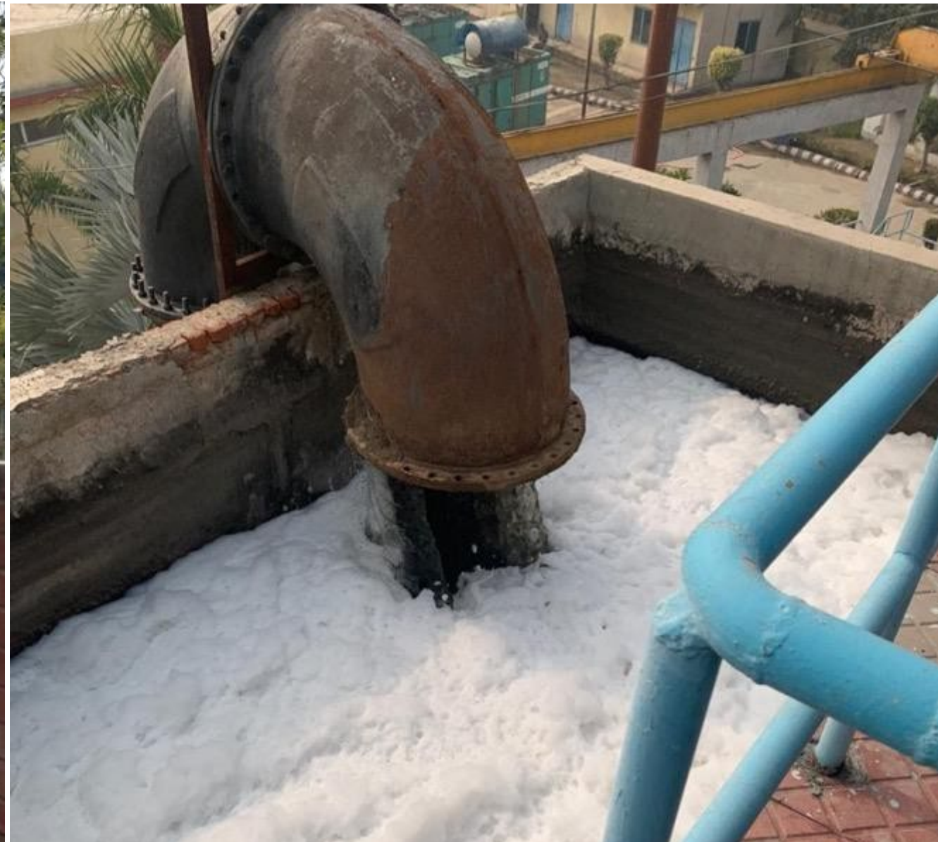
Photograph of inlet sewage
