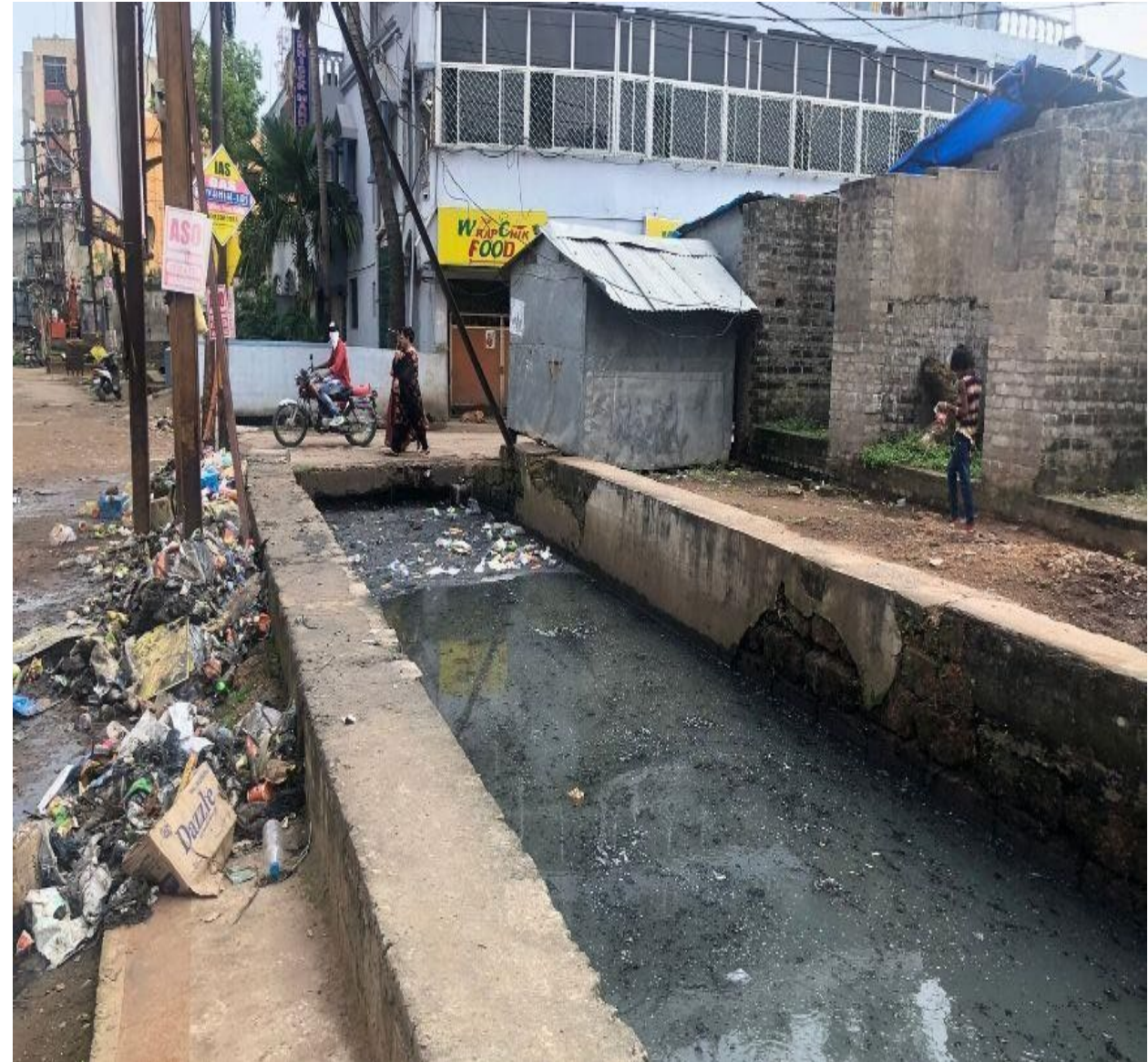
Photograph of SWD with visible/floating solids
